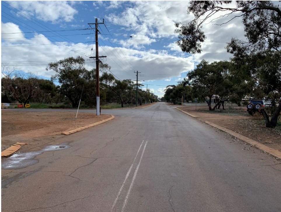
Figure 1: Broad Av looking west from approx. Slk 0.05 showing power pole prior to the CBH intersection (LHS) and damaged kerbing.
