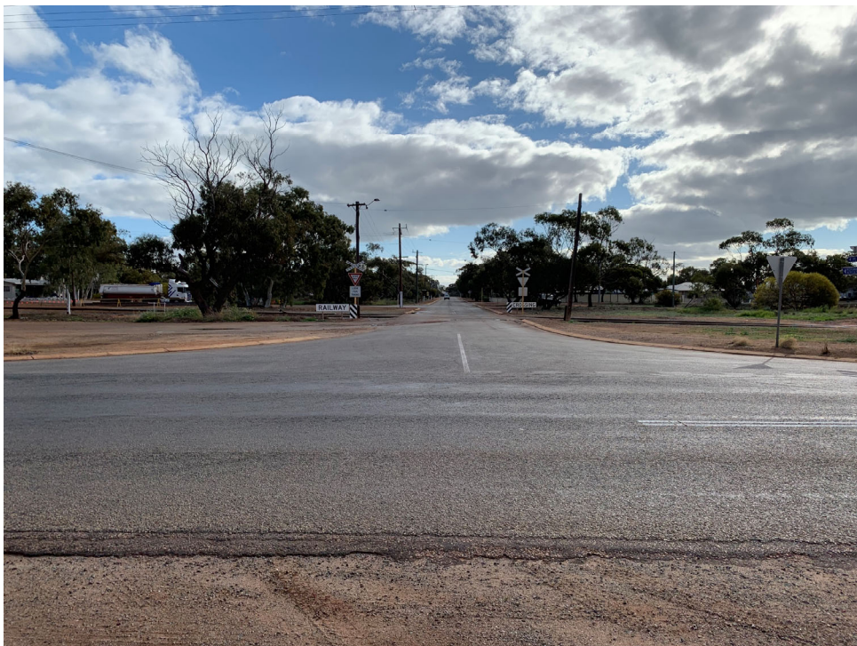
Figure 4: Broad Av looking west from Wubin Mullewa Rd intersection showing the CBH sampling station intersection (LHS), the rail spur line crossing and damaged kerbing on southern (LHS) side of intersection.
