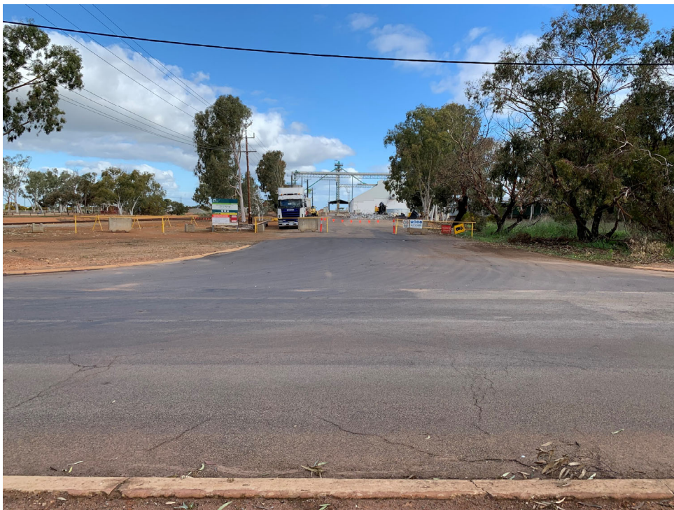
Figure 2: CBH entrance looking south from Broad Av showing kerbing removed on northern (RHS) side of intersection.
