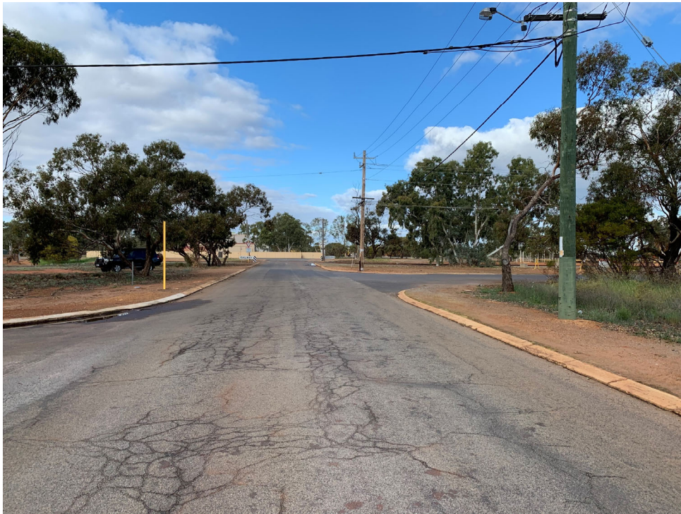
Figure 3: Broad Av looking east from approx. Sk 0.12 showing distressed surfacing.
